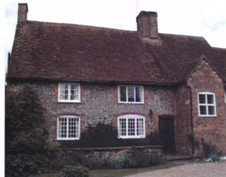
Fig. 14: Front (East) Elevation showing lack of corresponding joint
