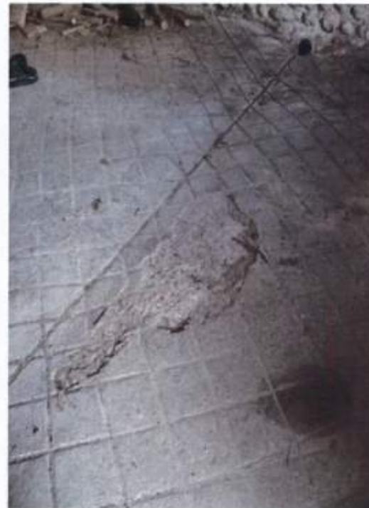
Fig.33: Existing grooved concrete floor to Stable showing deterioration
