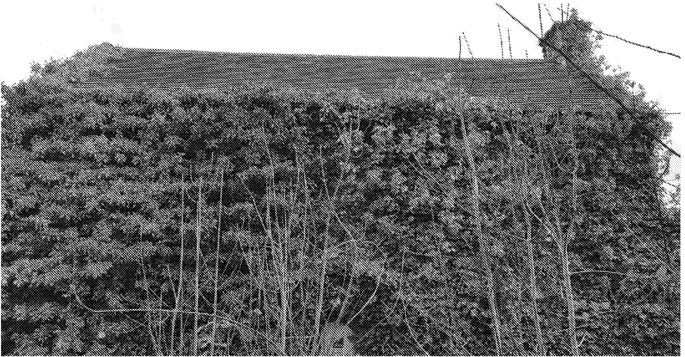
Photograph No. 3 - South of B2, showing the exposed, damaged tiles and heavy Ivy providing bat roost suitability.
