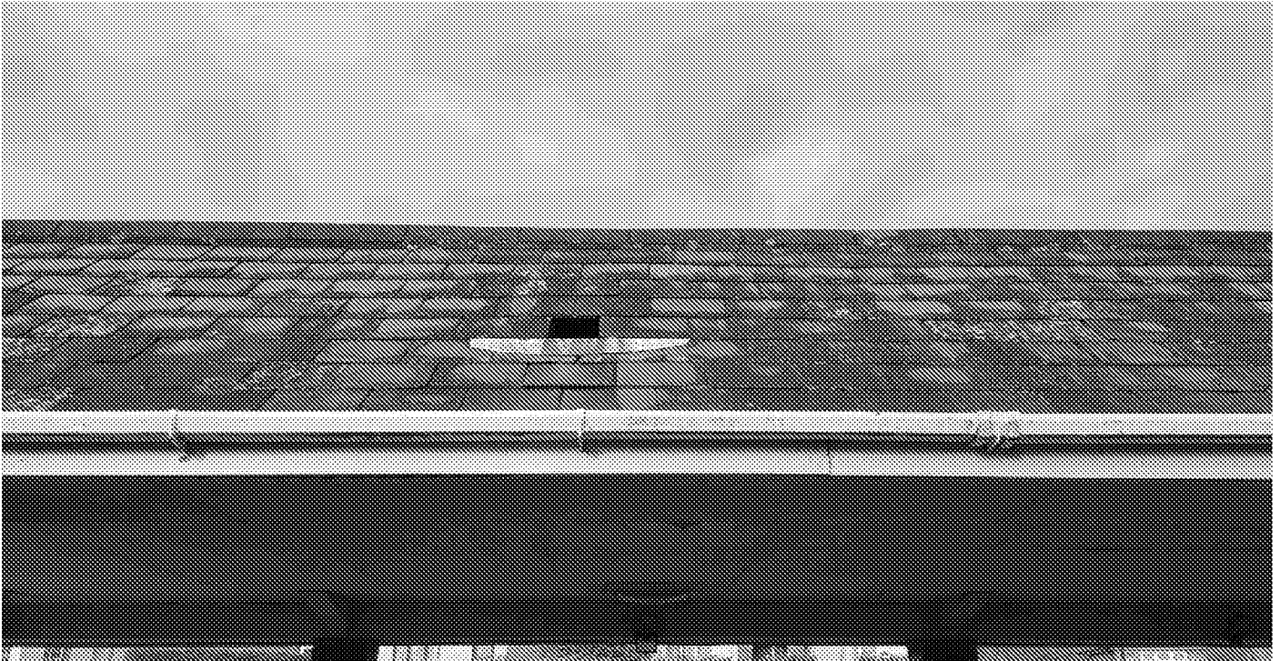
Photograph No. 5 - View of B3 (southern aspect) with exposed tiles and gaps under tiles providing bat roost suitability.
