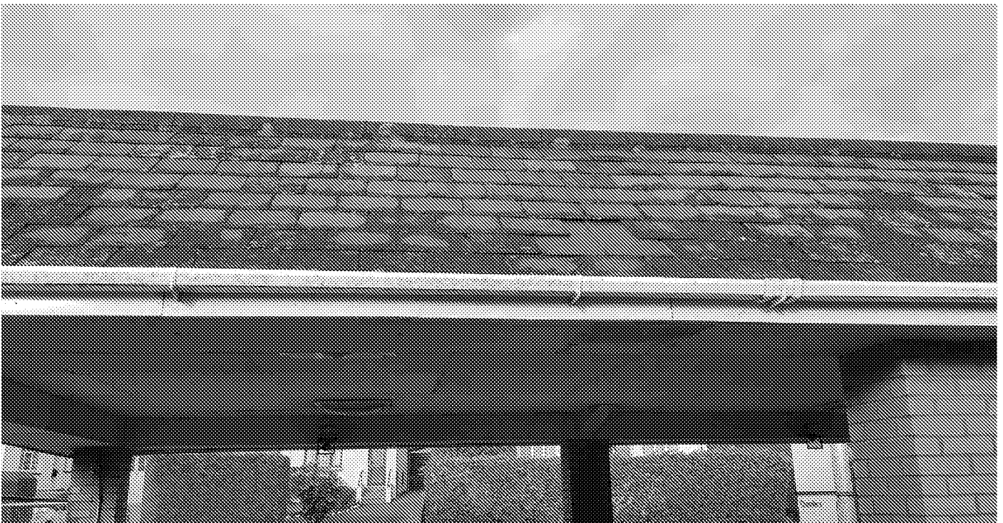
Photograph No. 6 - View of B3 (Northern Aspect) with exposed tiles and gaps under tiles providing bat roost suitability..
