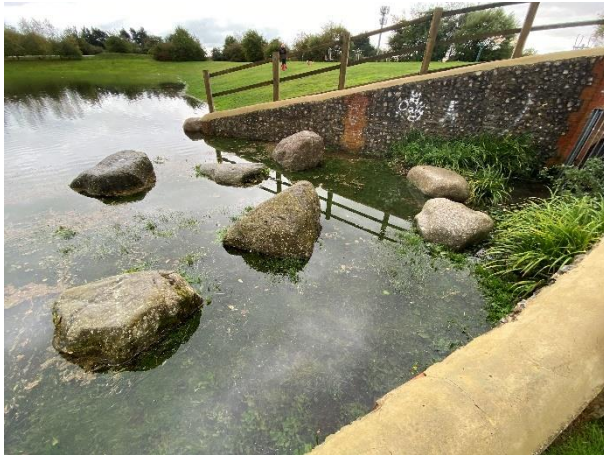
Photo 21: Large rocks and storm drain
