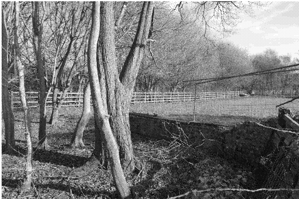
Plate 6: The remains of flint and mortar wall survive to the west of Brookenbee
