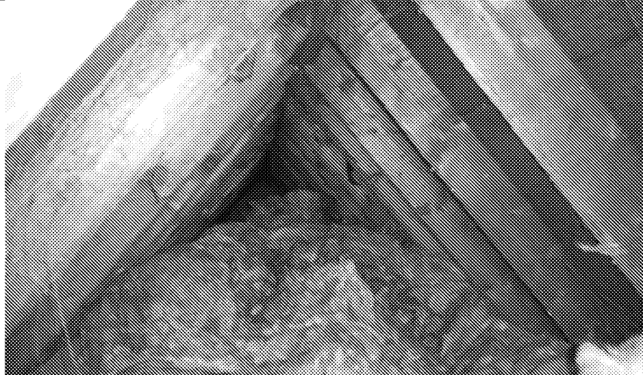
Photograph 5: The small void filled with insulation and dense cobwebs.
