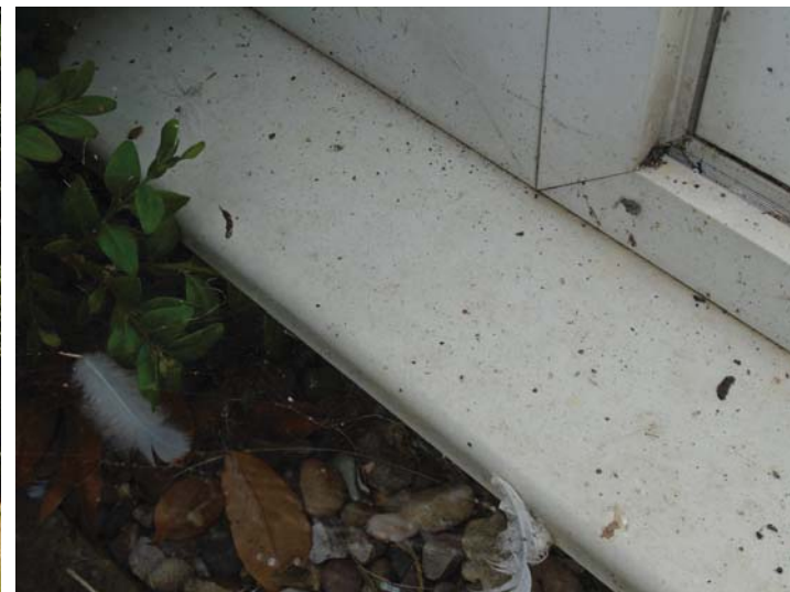
Bat droppings - building B1
