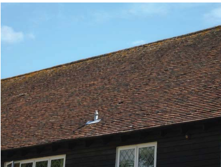
Building B1 - roof tile with gaps
