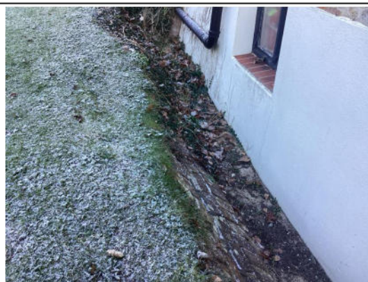
High external ground levels to the rear elevation
