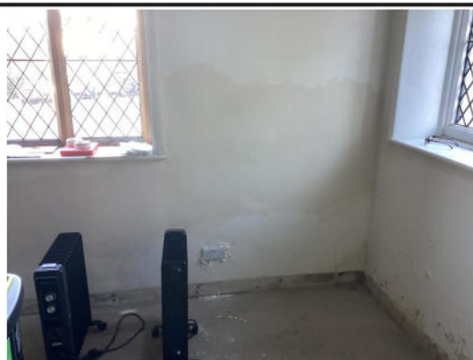
Further spoiling in first reception room
