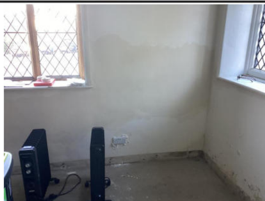
Further spoiling in first reception room
