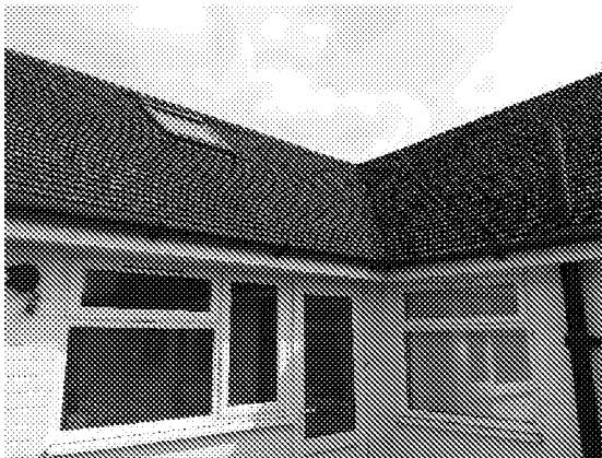
Plate 3. Western aspect of extension section of bungalow (B1) with gaps under tiles around window and in valley.
