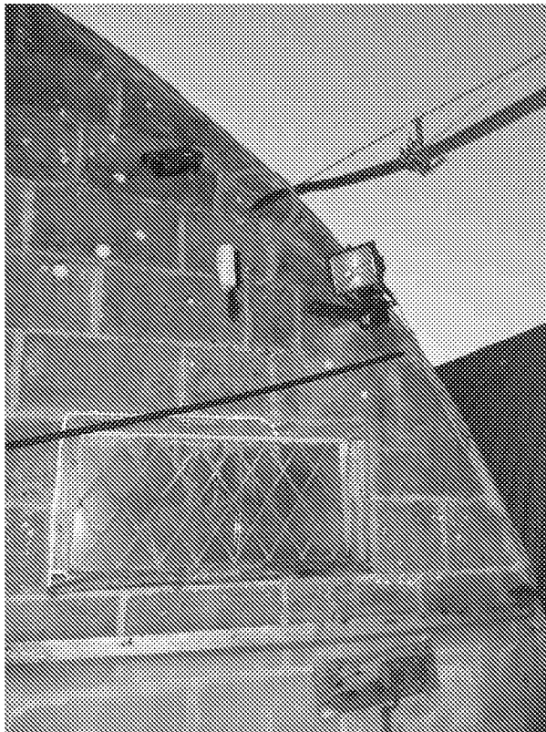
Plate 17. B4d showing hole in brickwork where soprano pipistrelle emerged in June 2018
