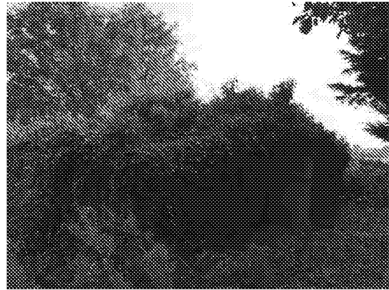
Plate 16. B13 – ivy covered dilapidated barn
