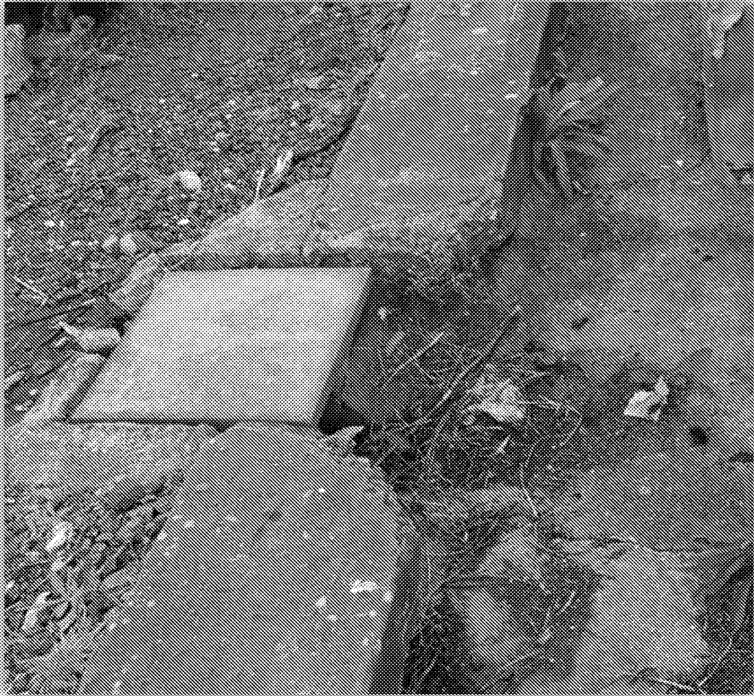
Image 3.2: Surface water drain outside a commercial unit
