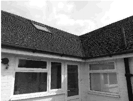
Plate 3. Western aspect of extension section of bungalow (B1) with gaps under tiles around window and in valley.
