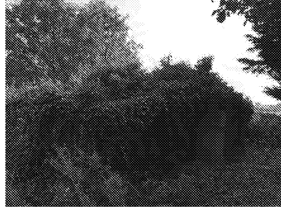
Plate 16. B13 – ivy covered dilapidated barn
