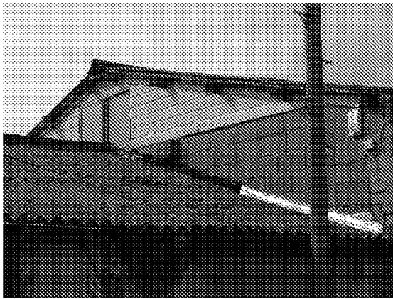
Plate 7. Wall between B2a and B2b showing gappy metal cladding.
