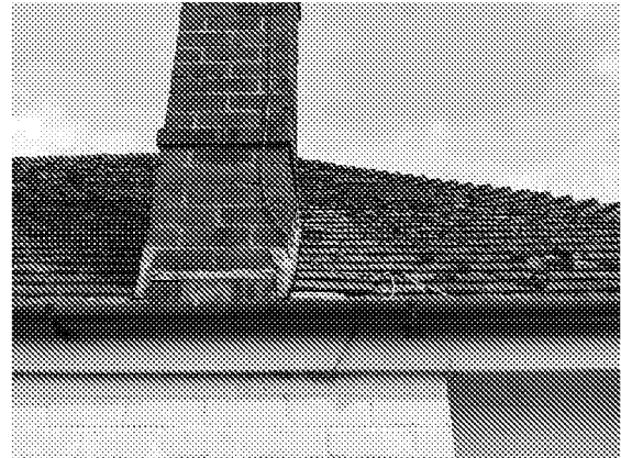
Plate 4. Northern aspect of bungalow (B1) with gaps under tiles around chimney.
