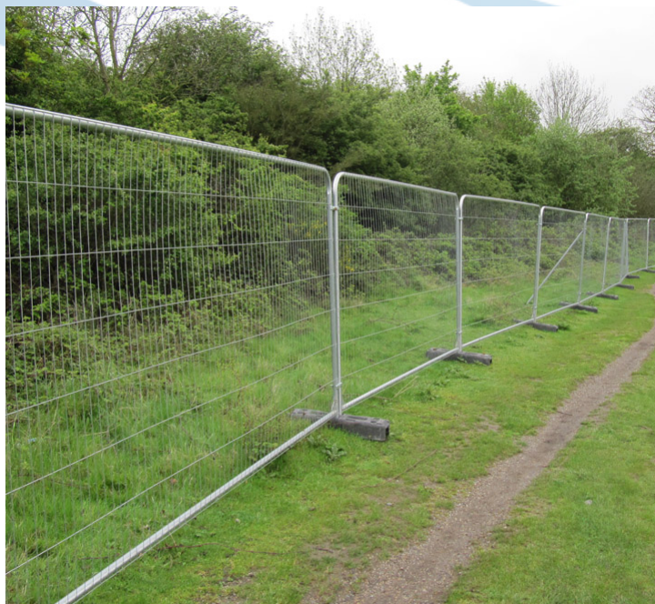
Anti Climb Heras fencing
