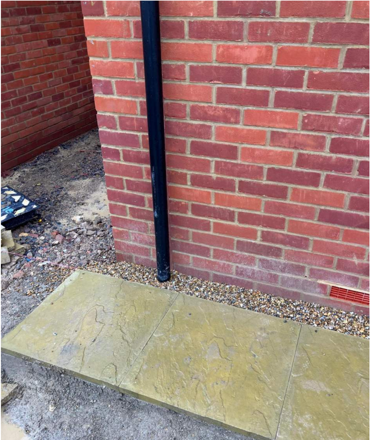
Photo of Rainwater Pipe Installed on Site
