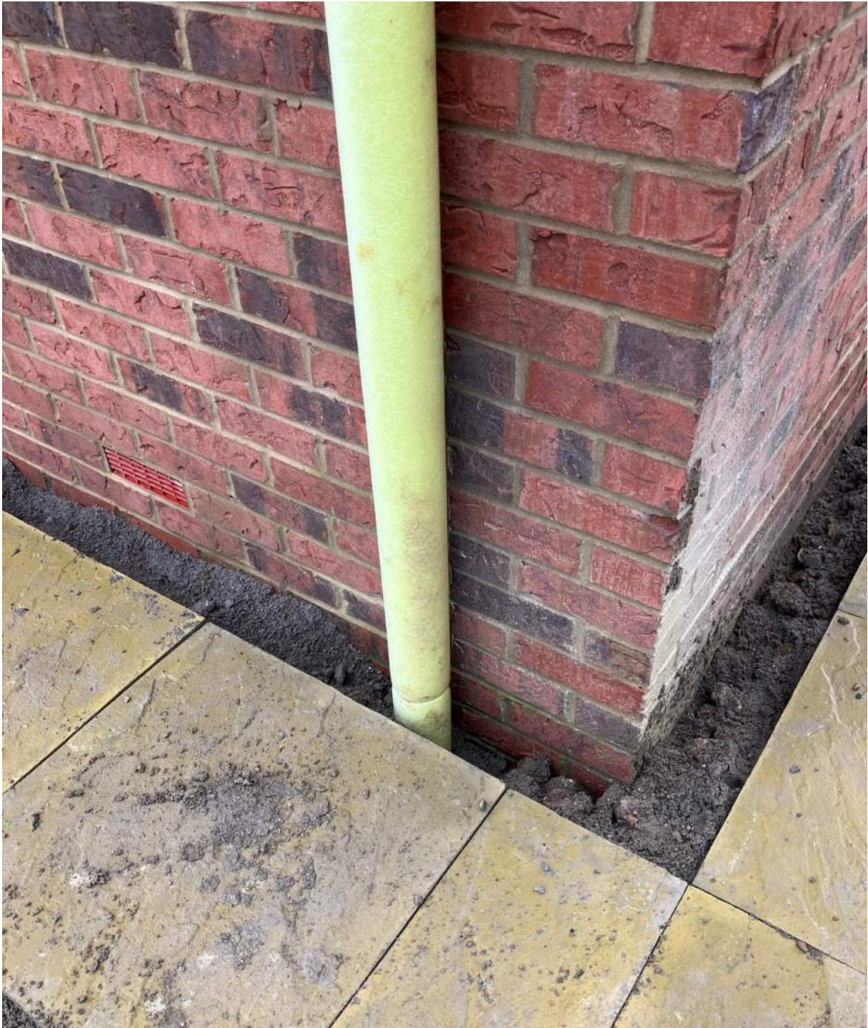
Photo of Rainwater Pipe Installed on Site
