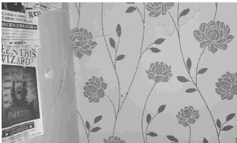
Photo 9 - Block A - crack in the return wall to the right of front bay window
