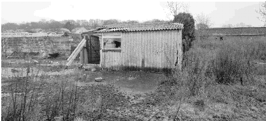
Photo 58 – Block G – Side view – Section of wall and roof missing
