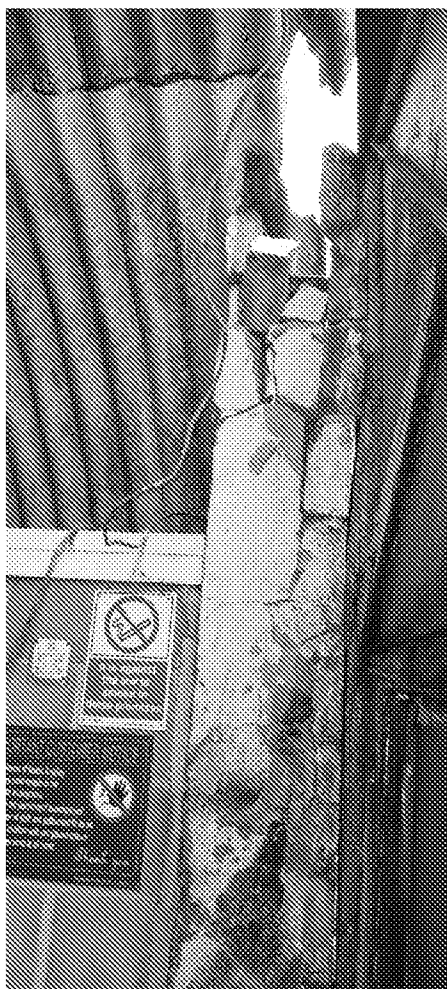
Photo 35 – Block C – Gable entrance of Hut C4 showing damage to the wall
