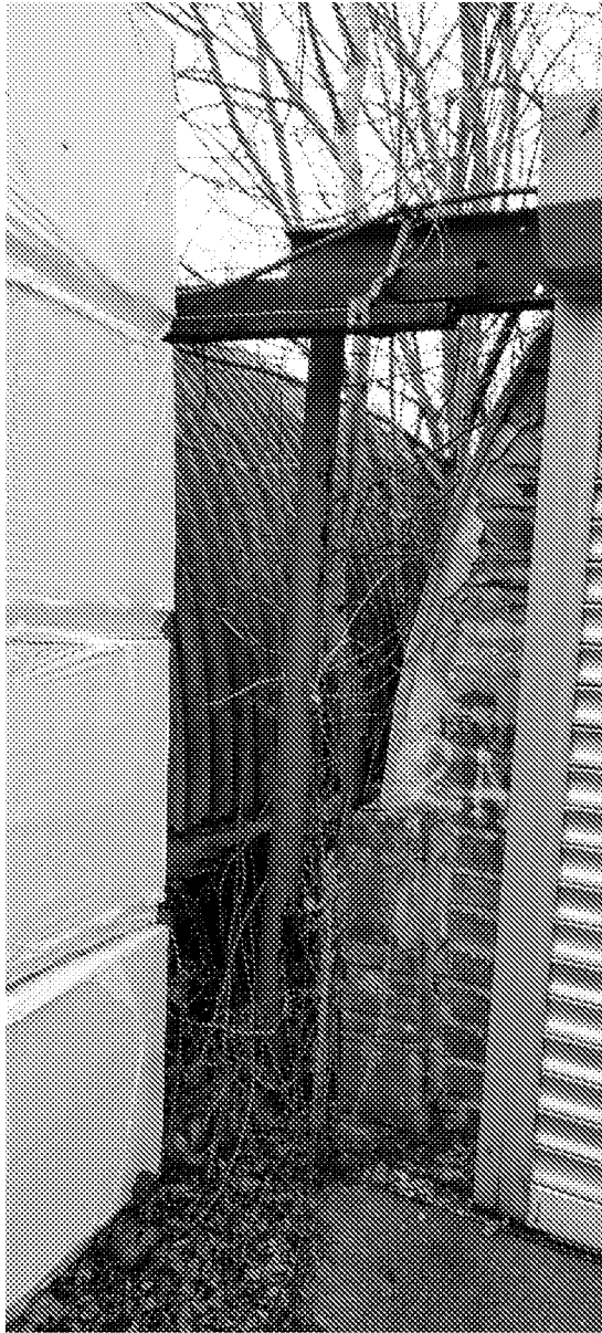
Photo 38 – Block C – Steel frame support to rear roller shutter door – The steel post is badly corroded
