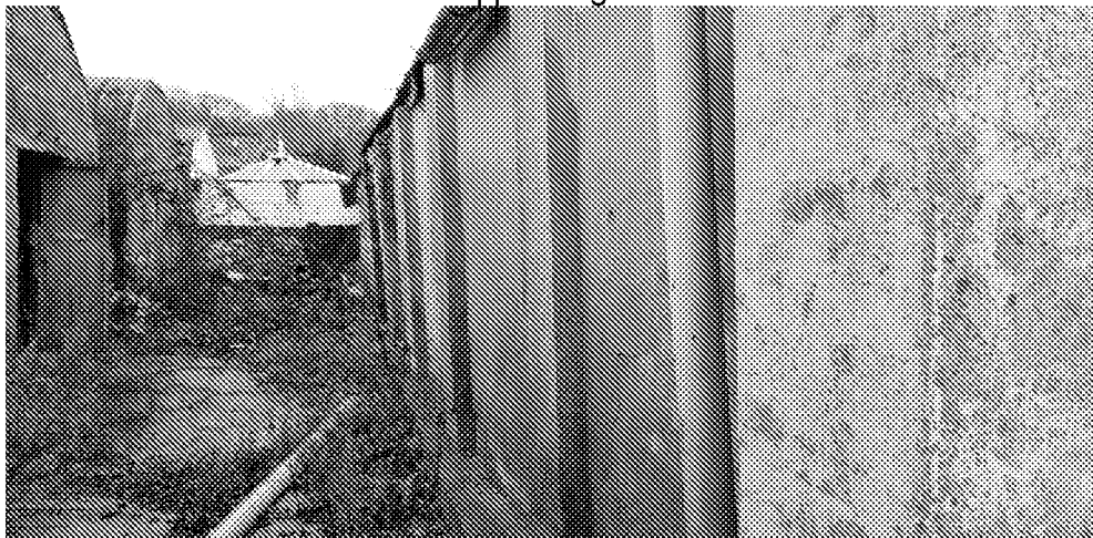
Photo 44 – Block D – View along side rear elevation showing wall leaning
