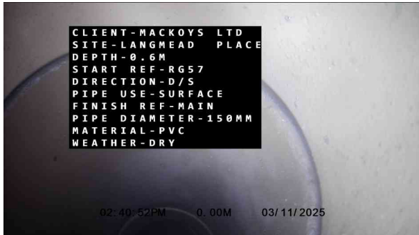
1, 00:00:00, 0.00 m Start node, gully, reference: RG57
