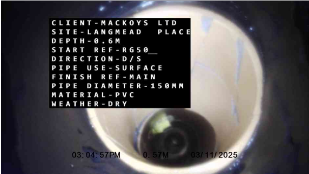
1, 00:00:00, 0.00 m Start node, gully, reference: RG50
