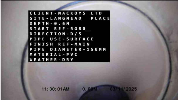
1, 00:00:00, 0.00 m Start node, gully, reference: RG80
