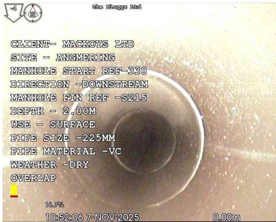
1, 00:00:00, 0.00 m Start node, manhole, reference: 330
