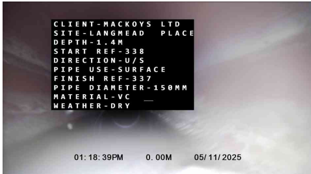
1, 00:00:00, 0.00 m Start node, manhole, reference: 338
