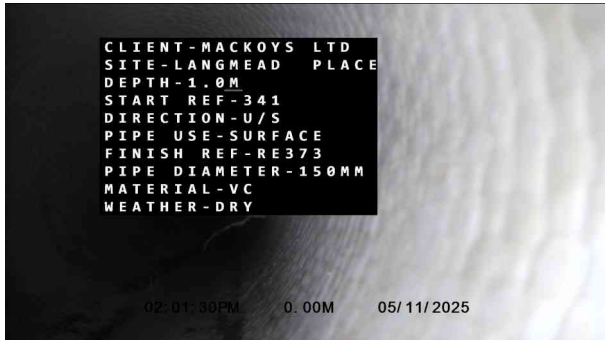
1, 00:00:00, 0.00 m Start node, manhole, reference: 341
