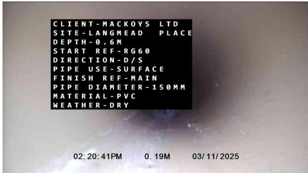
1, 00:00:00, 0.00 m Start node, gully, reference: RG60
