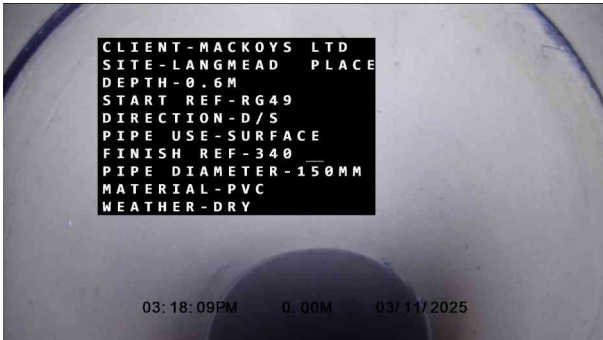
1, 00:00:00, 0.00 m Start node, gully, reference: RG49
