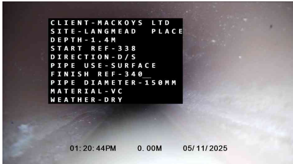
1, 00:00:00, 0.00 m Start node, manhole, reference: 338
