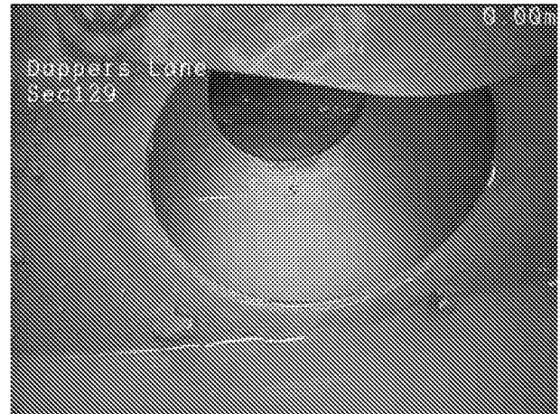
2, 00:00:33, 0.00 m Survey abandoned, Unable to cctv past hydrobrake
