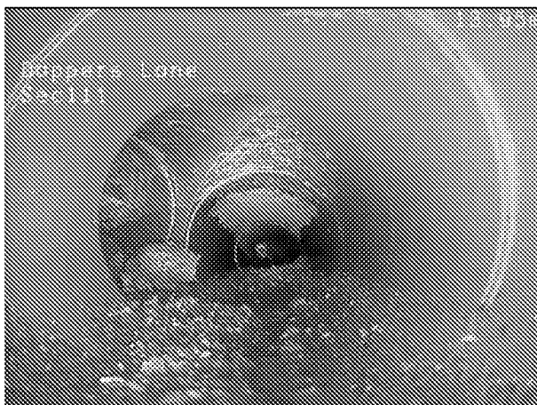
5, 00:02:04, 13.90 m Settled deposits, coarse, 15% cross-sectional area loss
