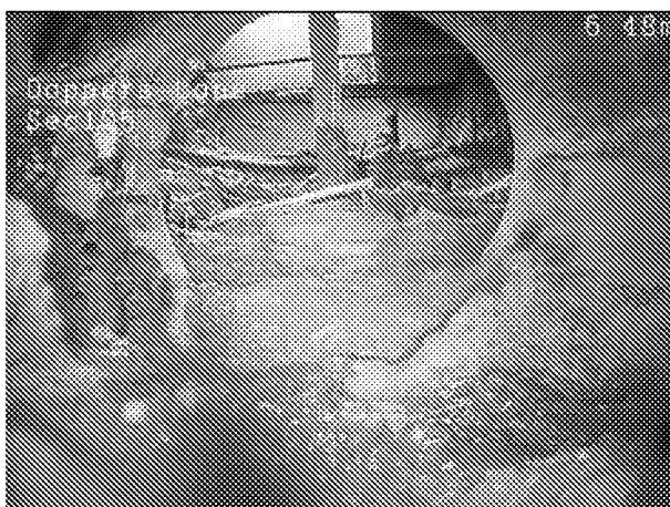
5, 00:00:41, 6.70 m Finish node, manhole, reference: RG, Debris in gully
