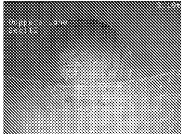
2, 00:00:15, 2.30 m Line deviates up
