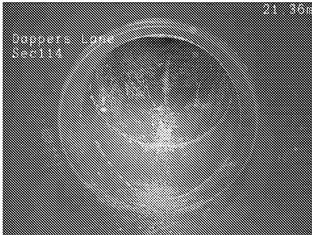
7, 00:01:15, 21.50 m Line deviates up
