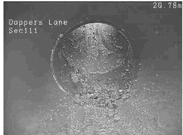
8, 00:01:27, 20.90 m Line deviates up
