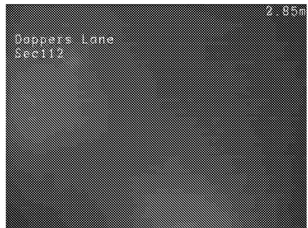
4, 00:00:29, 2.80 m Loss of vision, camera under water
