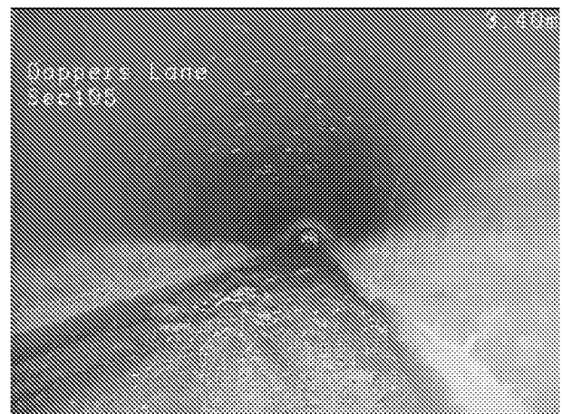
4, 00:00:20, 3.40 m Settled deposits, fine, 20% cross-sectional area loss, change
