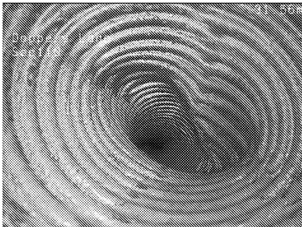
3, 00:02:07, 31.20 m Deformed sewer or drain, 40%
