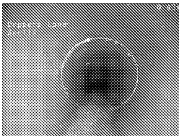
2, 00:00:14, 0.40 m Settled deposits, fine, 5% cross-sectional area loss
