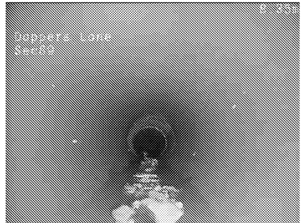
2, 00:00:33, 8.40 m Settled deposits, coarse, 10% cross-sectional area loss, start
