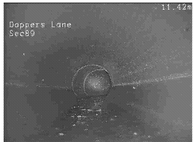
4, 00:00:50, 11.40 m Settled deposits, fine, 10% cross-sectional area loss, start
