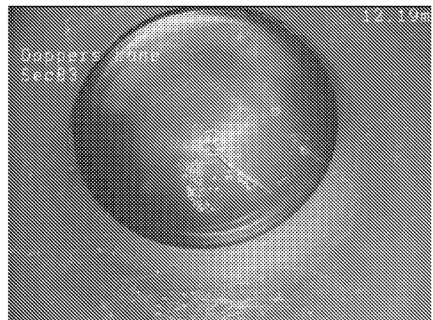
4, 00:00:57, 12.20 m Survey abandoned, Capped, rodding eye not installed
