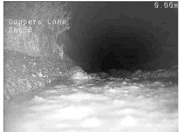
2, 00:00:00, 0.00 m Settled deposits, fine, 30% cross-sectional area loss, start
