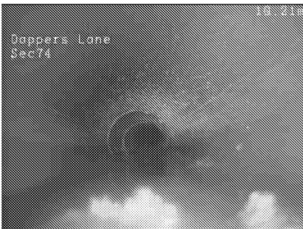
5, 00:01:00, 10.20 m Water level, 20% of the vertical dimension, Continuous
