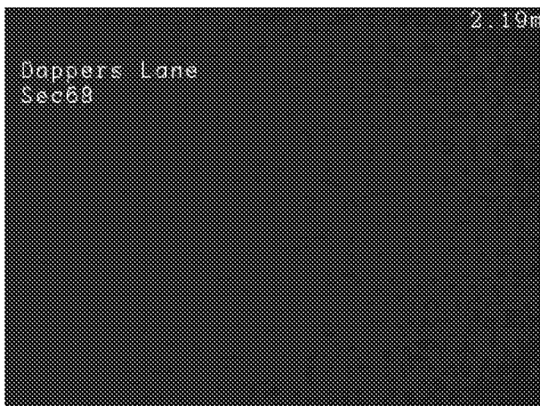
3, 00:00:26, 2.20 m Finish node, manhole, reference: RG, Road gully 100% full of debris
