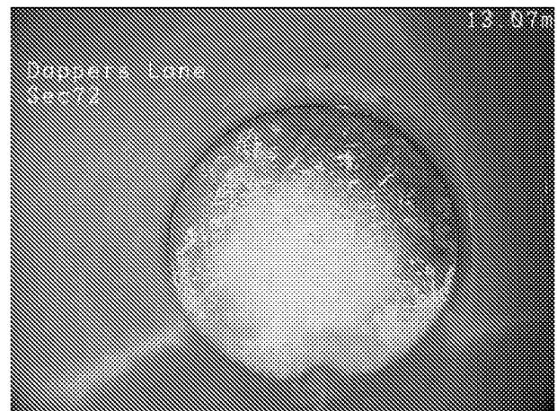
6, 00:01:21, 13.30 m Survey abandoned, Capped, rodding eye not installed
