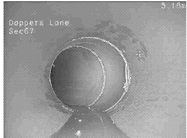
2, 00:00:55, 5.30 m Line deviates left
