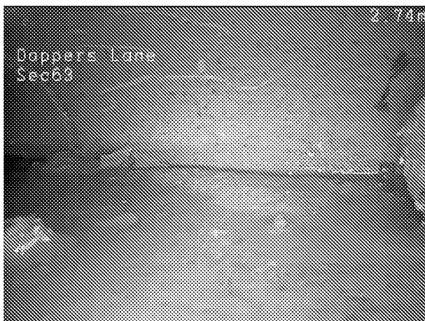
3, 00:00:40, 2.70 m Finish node, major connection without manhole, reference: JN, Heavy deposits in channel
