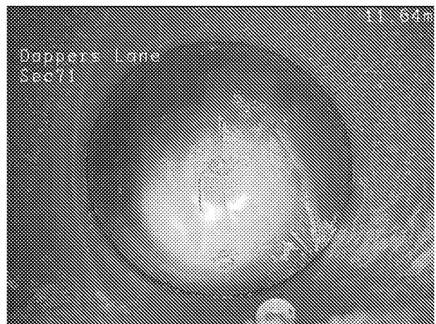
4, 00:00:39, 11.50 m Survey abandoned, Capped, rodding eye not installed
