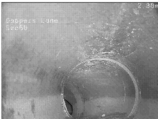
3, 00:00:30, 2.40 m Line deviates left
