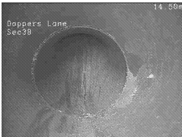
3, 00:00:44, 14.60 m Line deviates up
