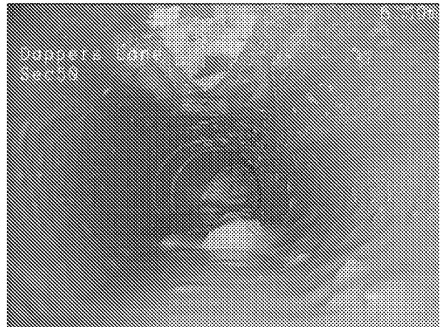
2, 00:00:36, 6.60 m Settled deposits, fine, 15% cross-sectional area loss, start
