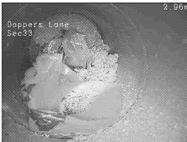
3, 00:00:25, 3.10 m Settled deposits, hard or compacted, 100% cross-sectional area loss, Concrete
