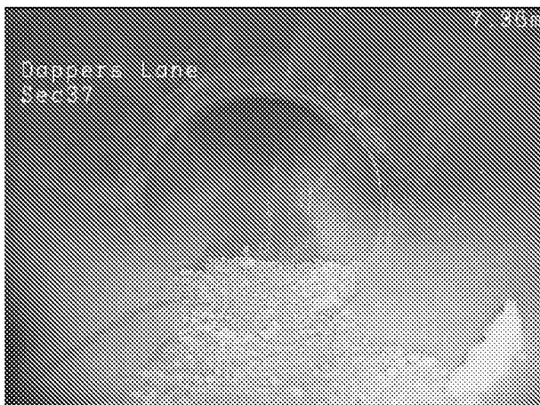
5, 00:01:22, 7.50 m Line deviates up
