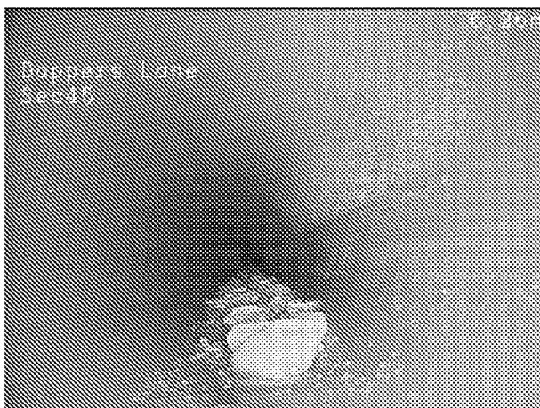
3, 00:00:38, 6.30 m Settled deposits, coarse, 20% cross-sectional area loss, start
