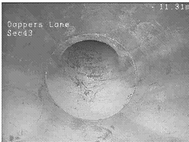
5, 00:00:47, 11.40 m Line deviates up
