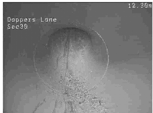
4, 00:00:52, 12.40 m Line deviates up
