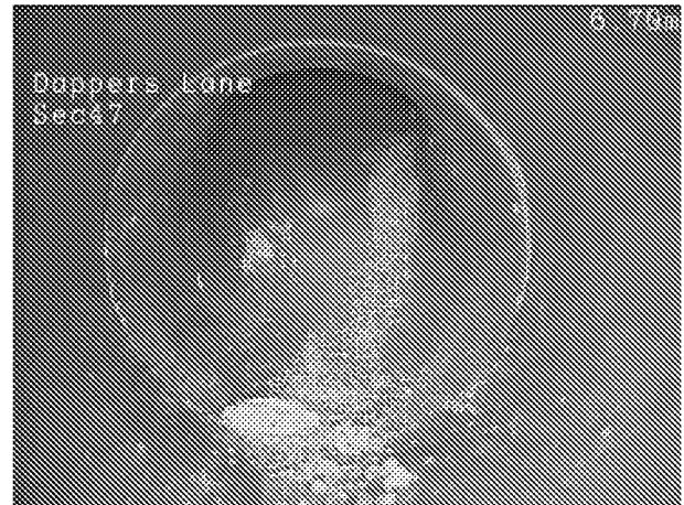
2, 00:00:31, 6.70 m Line deviates up
