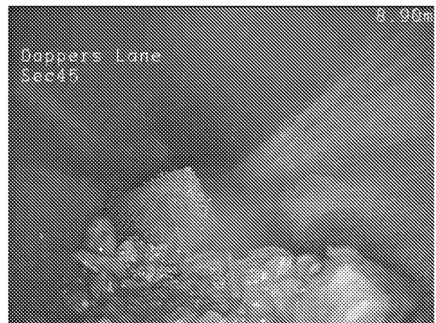
4, 00:00:02, 8.90 m Settled deposits, coarse, 50% cross-sectional area loss
