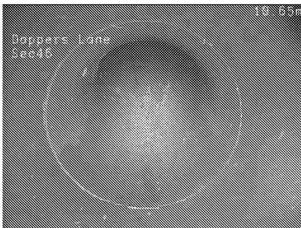
3, 00:00:53, 10.70 m Line deviates up
