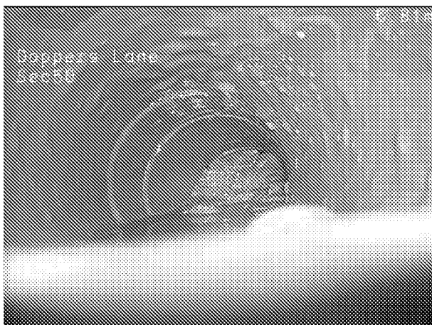
3, 00:00:40, 6.80 m Settled deposits, fine, 40% cross-sectional area loss, change
