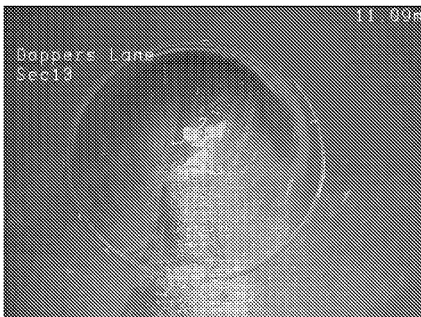
3, 00:00:45, 11.20 m Line deviates up
