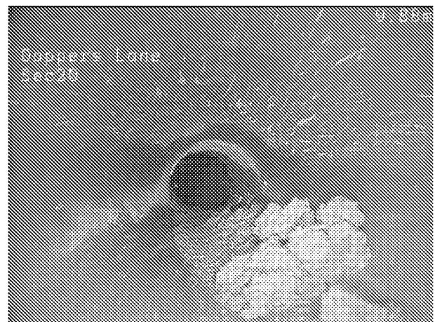
4, 00:00:49, 9.90 m Settled deposits, coarse, 20% cross-sectional area loss, start
