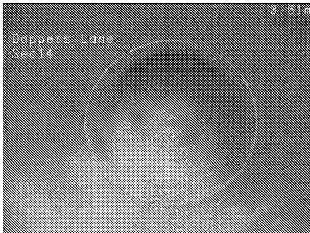
3, 00:00:22, 3.60 m Line deviates up
