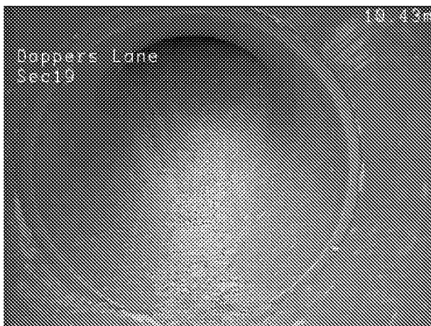
3, 00:00:57, 10.50 m Line deviates up
