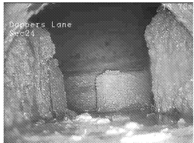
6, 00:00:53, 10.80 m Finish node, manhole, reference: F1, Debris in channel
