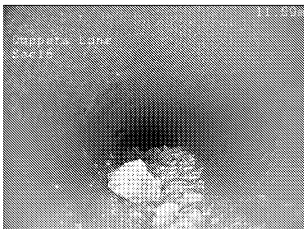
5, 00:00:53, 11.20 m Settled deposits, coarse, 30% cross-sectional area loss, start
