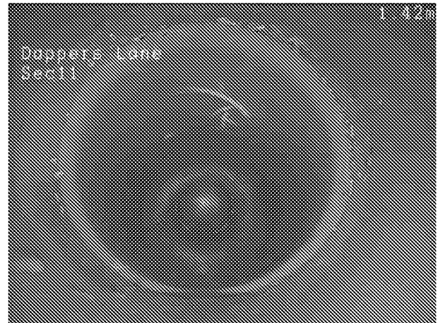
2, 00:00:20, 1.50 m Pipe material changes to vitrified clay at this point
