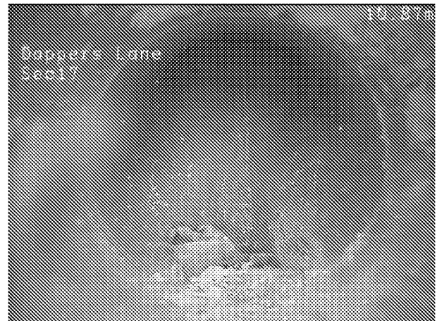
4, 00:01:18, 11.00 m Line deviates up
