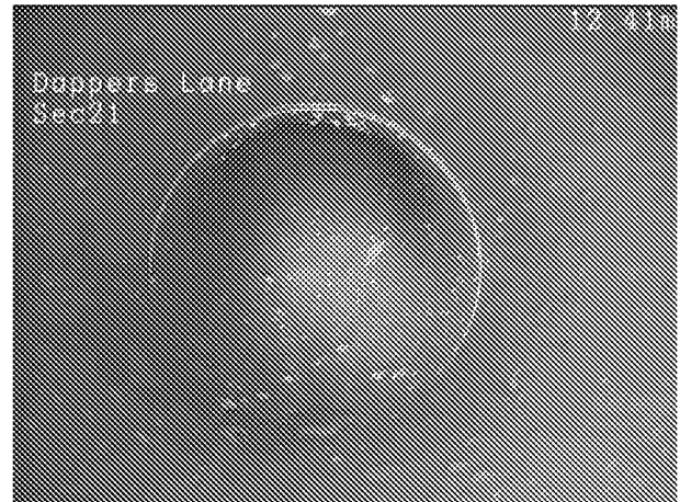
2, 00:00:41, 12.50 m Line deviates up
