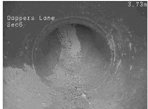
2, 00:00:24, 3.80 m Line deviates up
