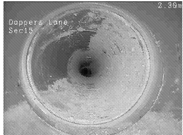
2, 00:00:19, 2.30 m Line deviates up
