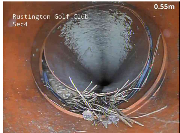
4, 00:00:18, 0.70 m Joint displaced, large
