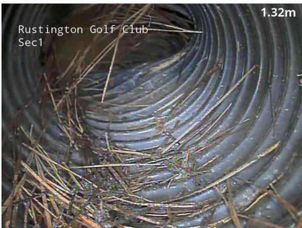
5, 00:01:15, 1.40 m Deformed sewer or drain, 50%
