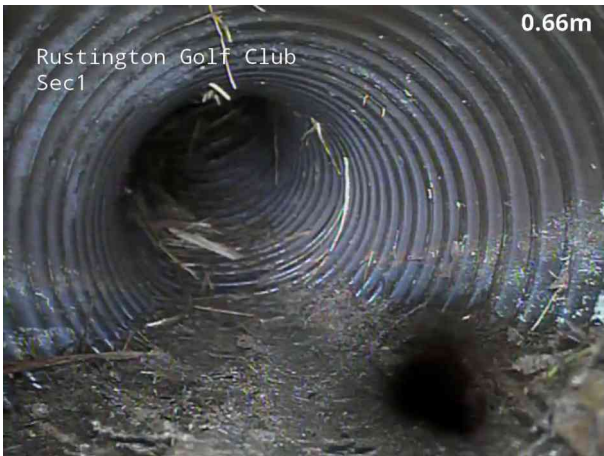
3, 00:00:32, 0.80 m Line deviates up
