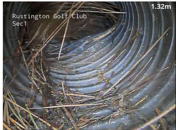
4, 00:01:15, 1.40 m Deformed sewer or drain, 50%
