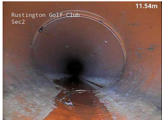
4, 00:00:44, 11.70 m Joint displaced, medium
