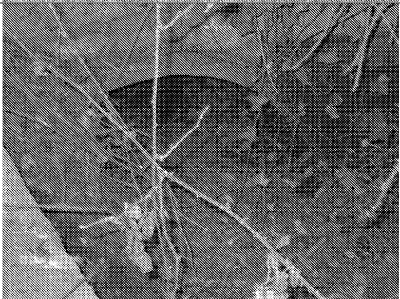
Photo 6: View of one of the pipes in the south west corner where mammal digging was detected
