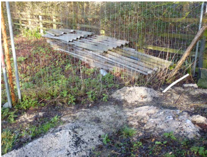
5 Possible ACM sheets.
