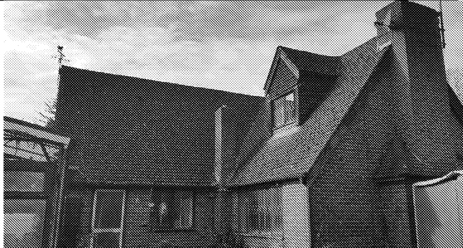
Photograph 2: The back of the house with flush tiles but slightly warped weatherboarding.
