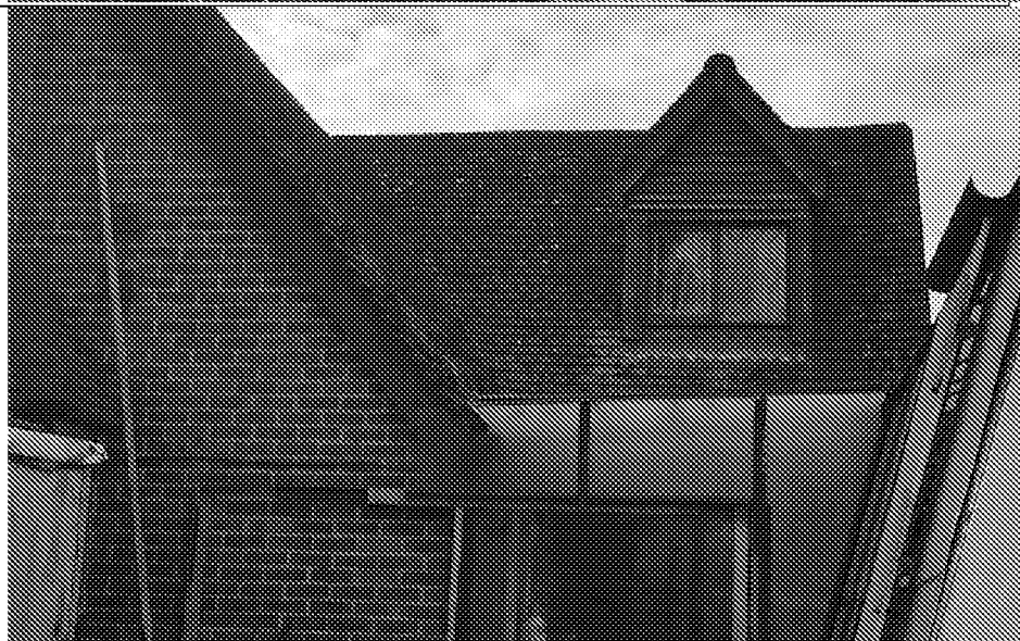
Photograph 3: The back of the house again with flush tiles but some warped weatherboarding.
