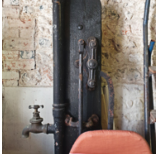
Old pump in outbuilding
