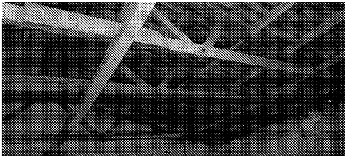
Photo 20 – Block B- Roof truss propped by timber beam
