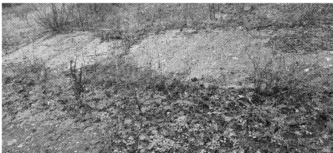
Photo 64 – Adjacent to Block E - Isolated ground bearing slab
