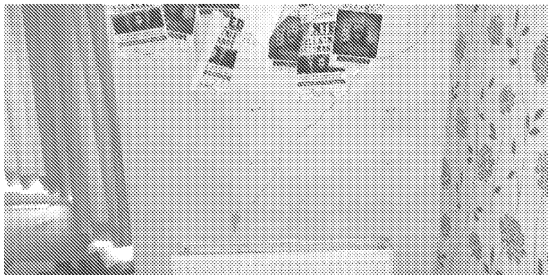
Photo 6 - Block A – crack in wall to the right of the of front bay window
