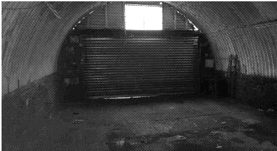
Photo 37 – Block C – Roller shutter door at the rear gable
