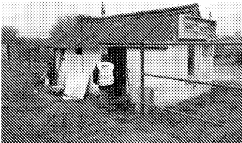
Photo 56 – Block F – View of the building. The cable ducts are visible outside.
