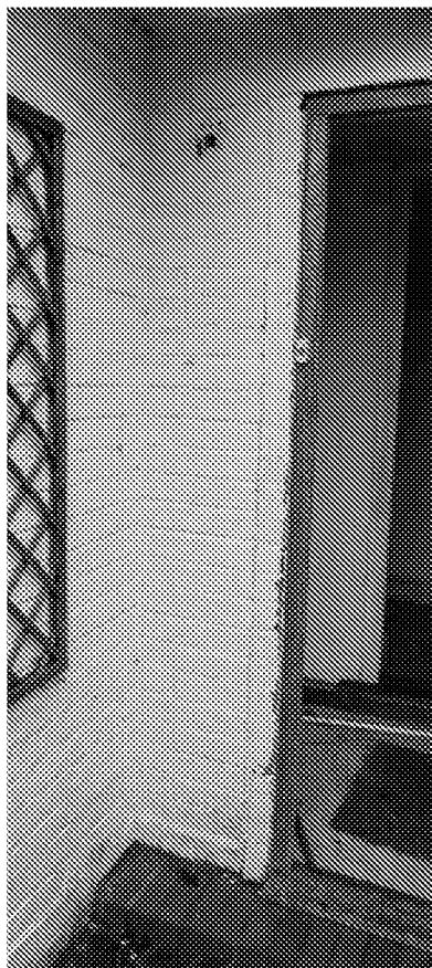
Photo 13 - Block A – Front elevation - cracking at the front door
