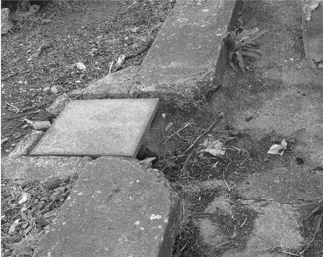
Image 3.2: Surface water drain outside a commercial unit
