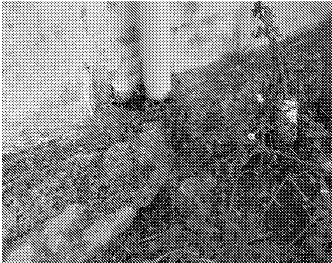
Image 3.1: Downpipe from commercial units
