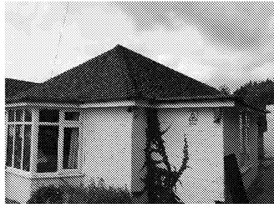
Plate 2. Southern and eastern aspect of bungalow (B1) with missing mortar under hip tiles.
