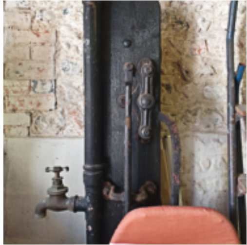
Old pump in outbuilding
