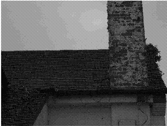
Photo 5: The cottage with gaps under the tiles.
