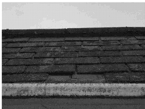
Photo 2: The missing roof tiles on the carport.
