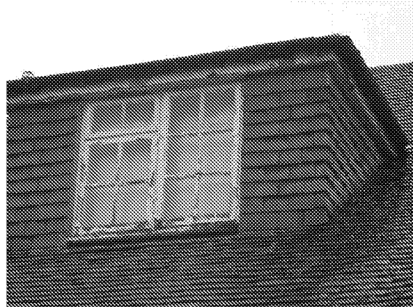
Photo 6: The dormer window on the cottage with loose hanging tiles.
