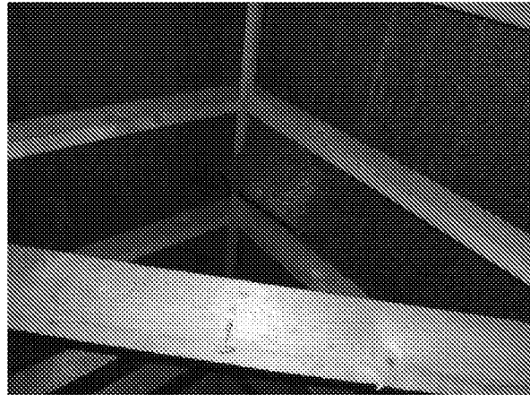
Photo 4: The loose bituminous lining in the loft of the cottage.
