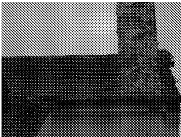
Photo 5: The cottage with gaps under the tiles.
