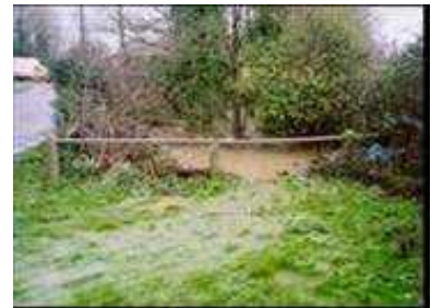
Entrance to Weavers Hill culvert overflowing onto Water Lane
