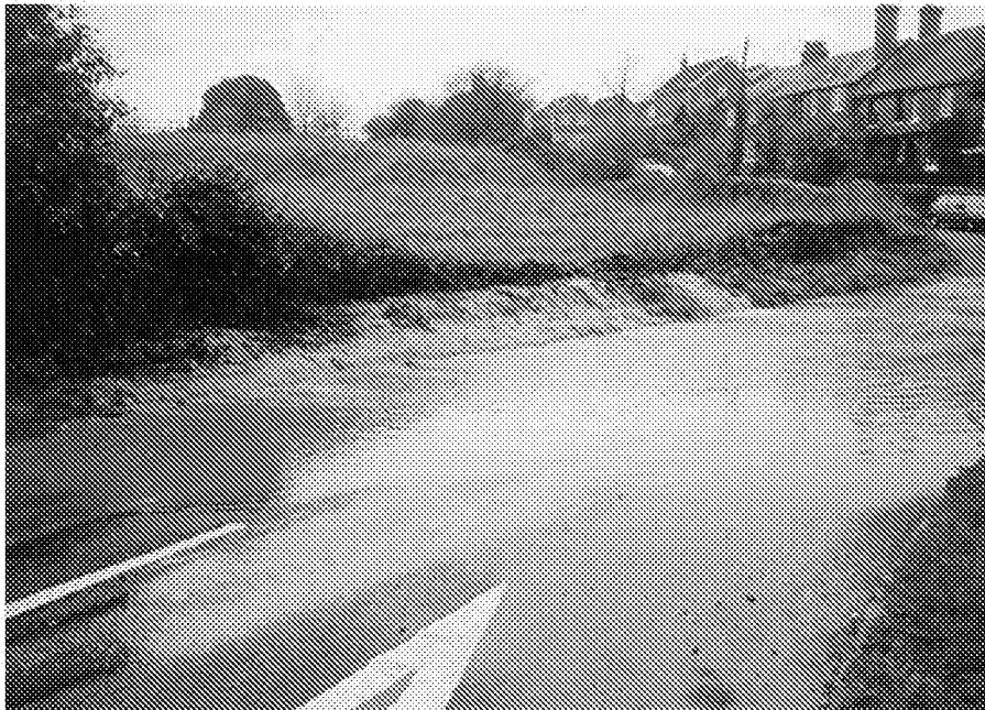
This photograph below shows water escaping from a manhole on the inadequate highway culvert through which the Black Ditch flows downstream of the development site.
