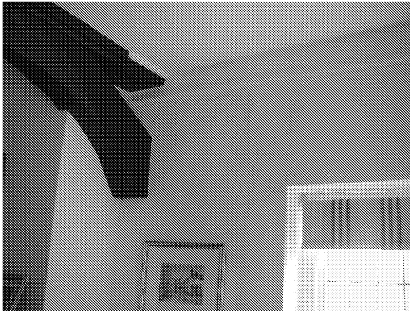
Photo – Damp ingress stains to internal wall (taken July 2015).
