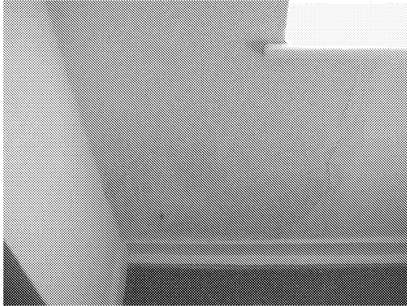
Photo – More damp staining on the inside of the wall.
