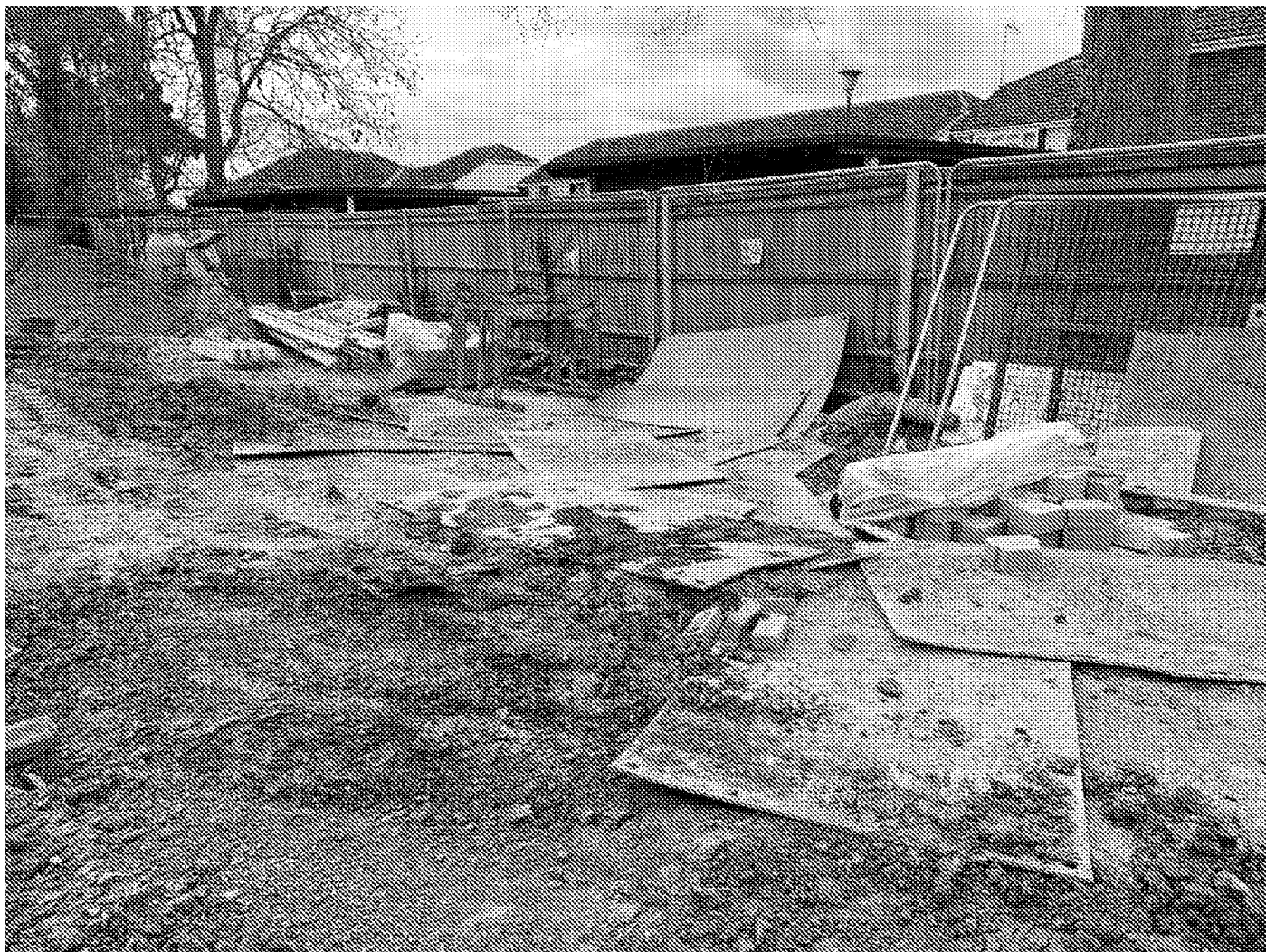
Fig.2. Looking south-west across exposed RPA of T04 showing deliberate misplacement of unsecured ground protection mats and stored materials within.
