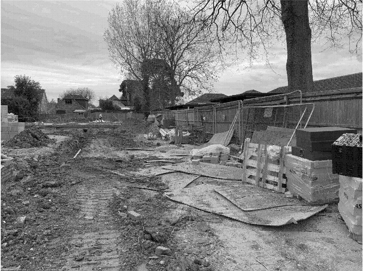
Fig.1. Looking south from near site entrance. T04 Turkey oak (TPO) to the right of frame, in the grounds of Malmayne Court. Note service run (open excavation with grey plastic duct visible) and tracked vehicle marks.
