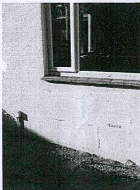
Photo 3 – External cracking below the window.
