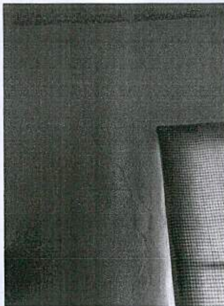
Photo 2 – Vertical cracking adjacent to window.
