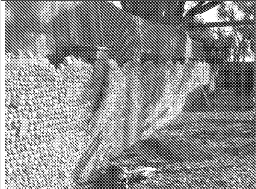
Picture 3. Retaining wall in proximity to T1-T3 with significant lean and cracking
