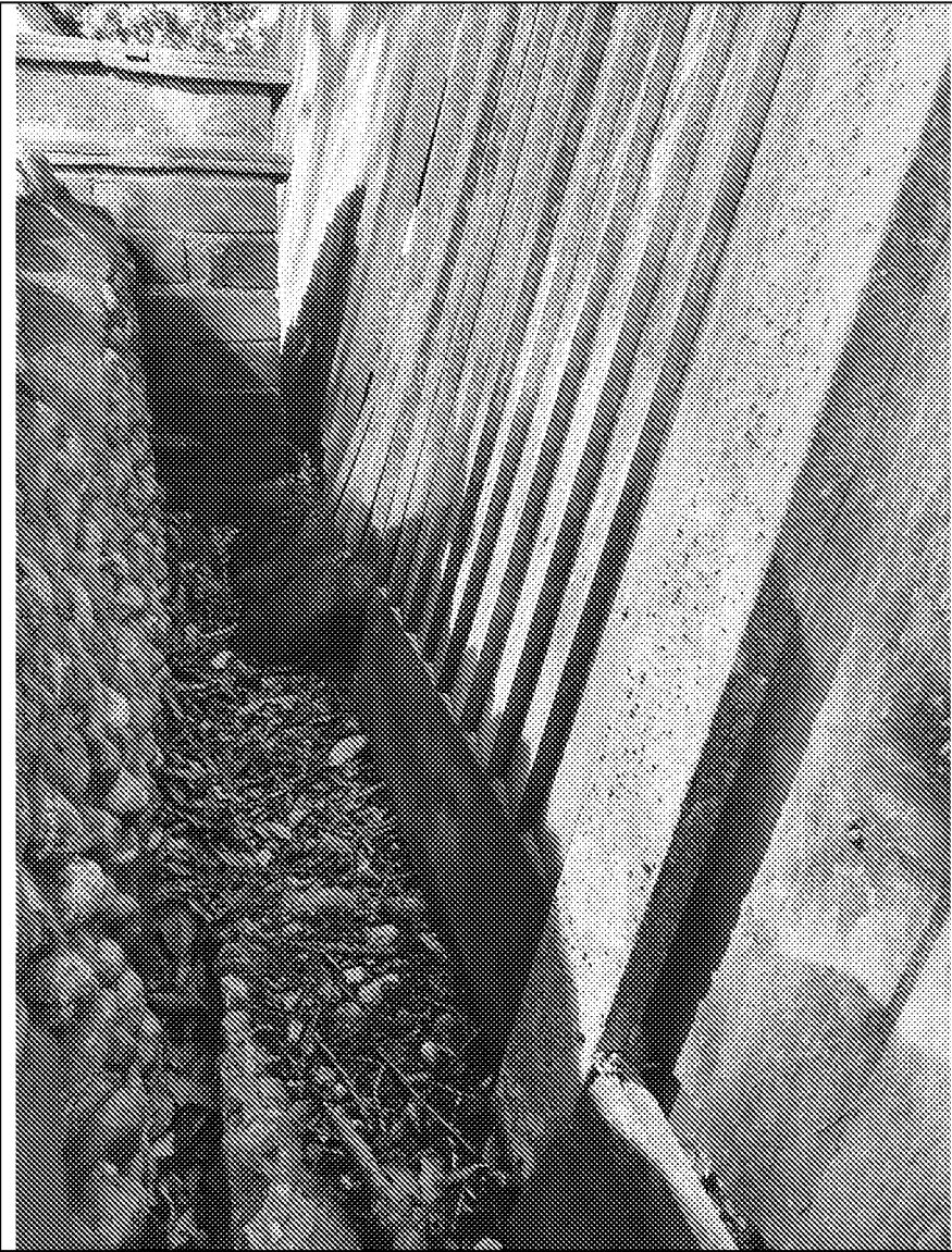
Picture 4. T1 roots in concrete with wall pillar.
