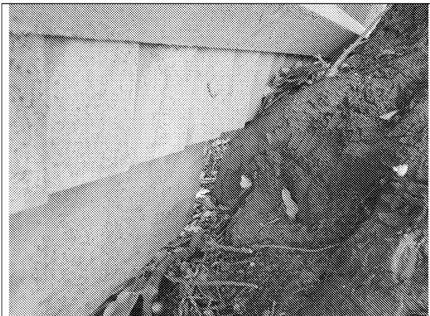
Picture 5. T3 roots in concrete with wall pillar.
