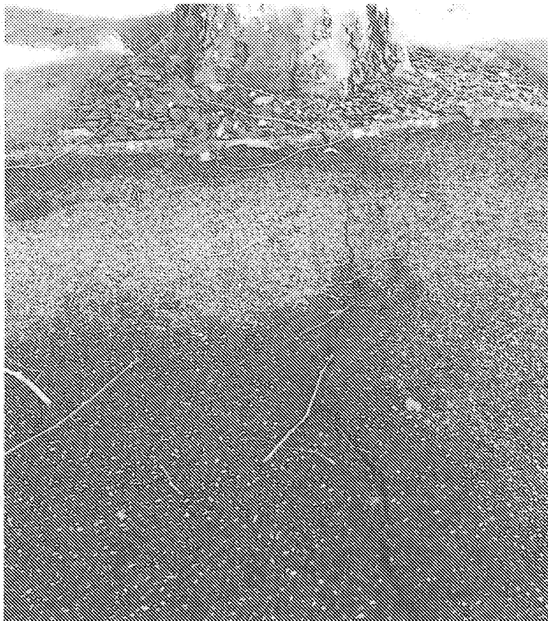
Damage to the drive; picture does not show the amount of ground heave clearly but it is considerable.
