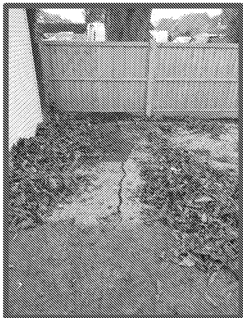
Picture 5 – T1 Horse Chestnut viewed from #2 with cracking of concrete
