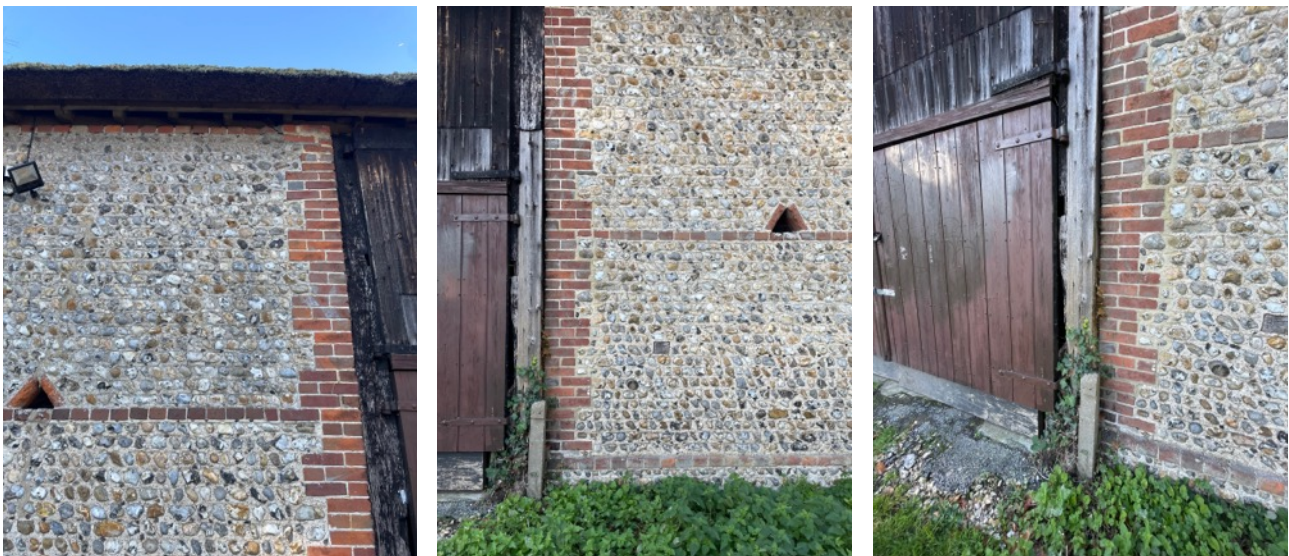
fig 2-4 Localised areas requiring minor repairs.
