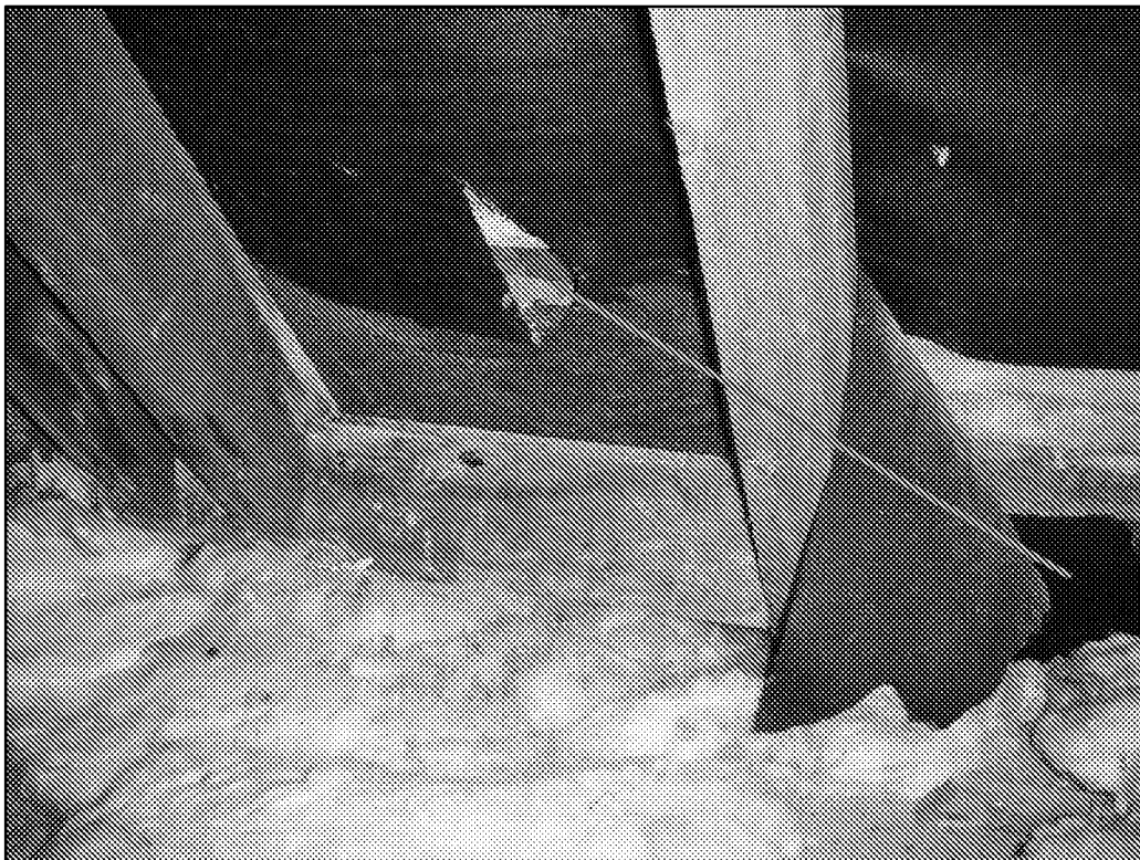
Photograph 2. Showing torn roof lining in V2.
