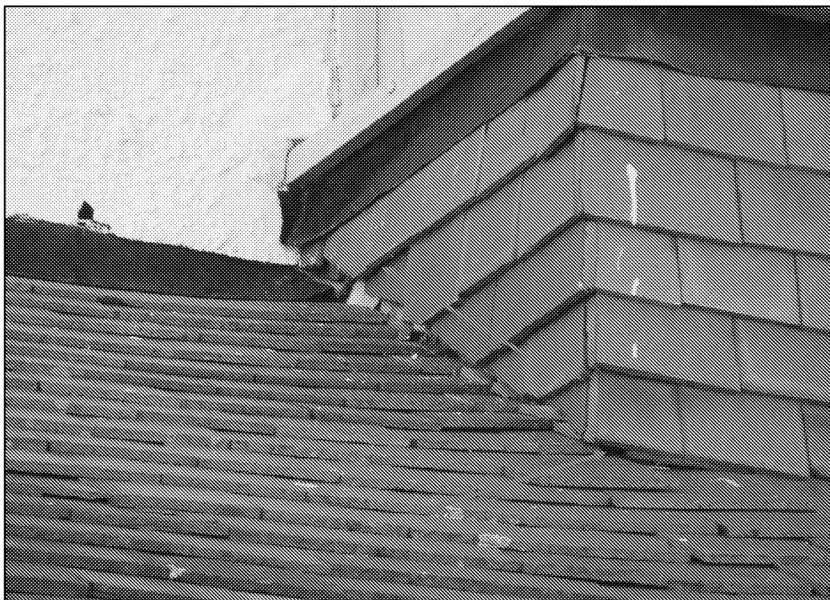
Photograph 4. Gaps associated with hanging tiles on Building A.
