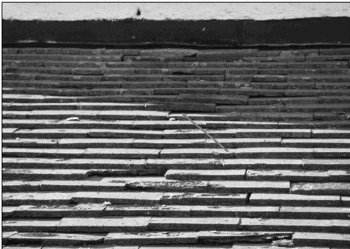
Photograph 3. Showing gaps under missing, broken and lifted roof tiles on Building A.
