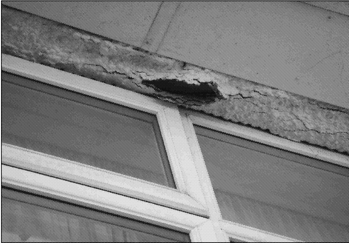
Photograph 5. Showing hole in render between wall and soffit on the north elevation of Building A.
