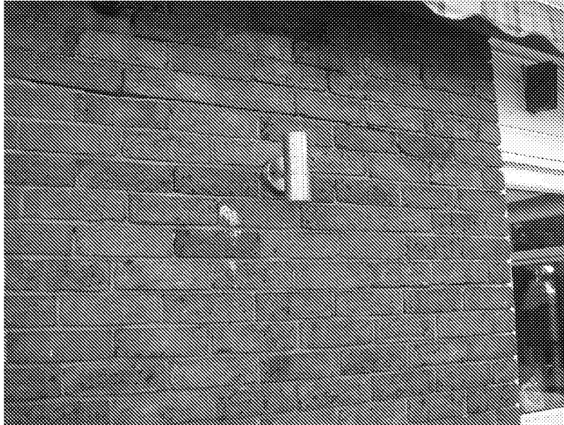
Pic – some of the deteriorated brickwork.
