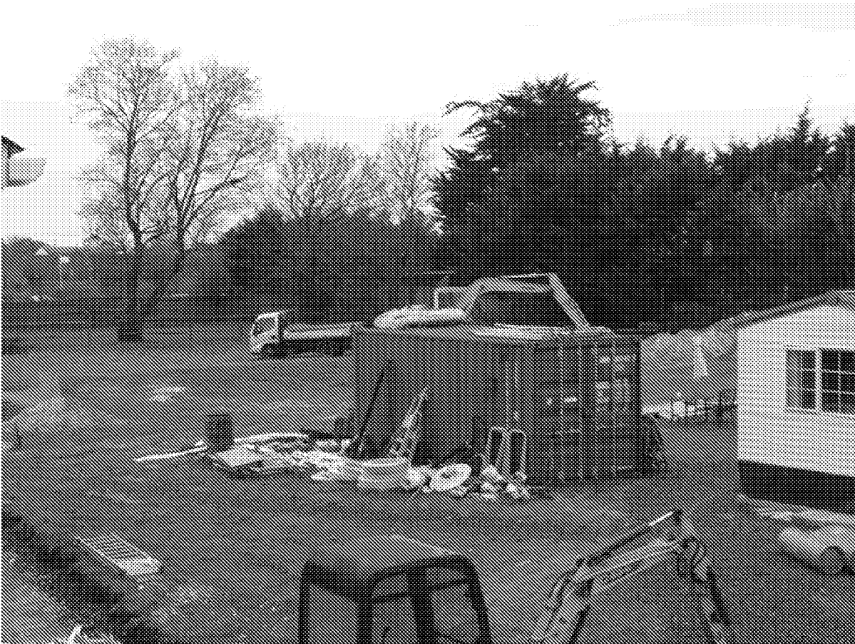
In this photo you can't actually see the 14 gas bottles littering the site. (We have had up to 19 in the past and there are 14 again now)
