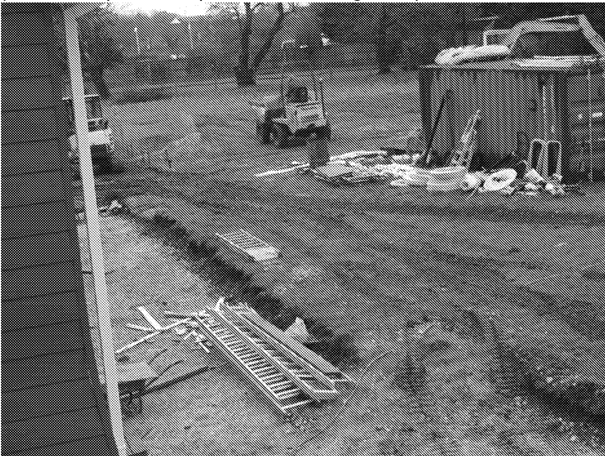
This work being done now, is actually on the middle site of three. They have never been properly fenced off from each other and we were forced to pay for the only fence which exists on the site, to separate us
