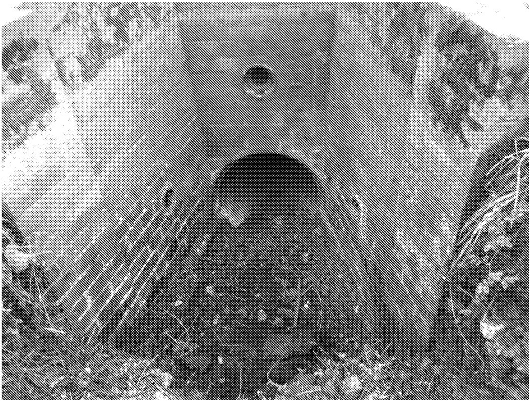
Land Drain Railway Culverts (approx. 450 mm to 600 mm Ø)
