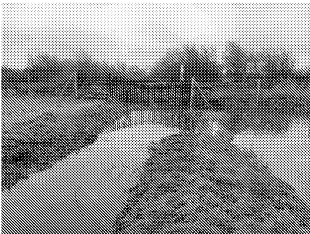
Photograph 6 – Flooded access onto railway line along southern boundary of the Site
