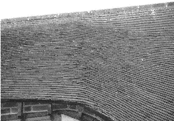
Gaps under roof tile on 'eyebrow' roof, E side, B1
