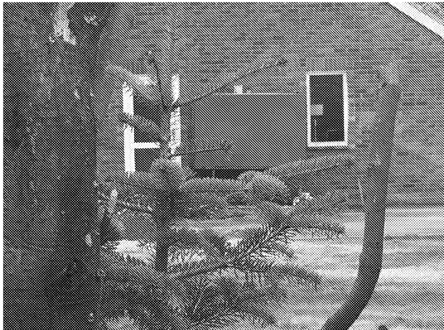
Photograph 13: View of the heating oil tank adjacent to the property to the south of the site
